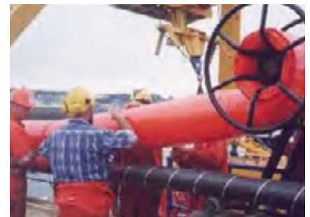
2. SeaSerpent being attached to the HVAC cable showing Seaflex manual brake RDS.
