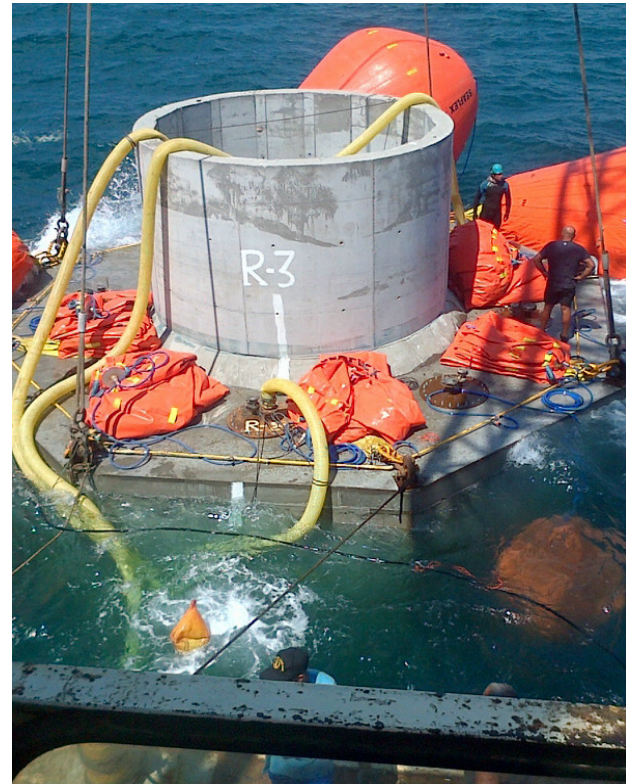
Sinking of Intake Tower (note submerged lower tier of buoys as upper tier is inflated)
