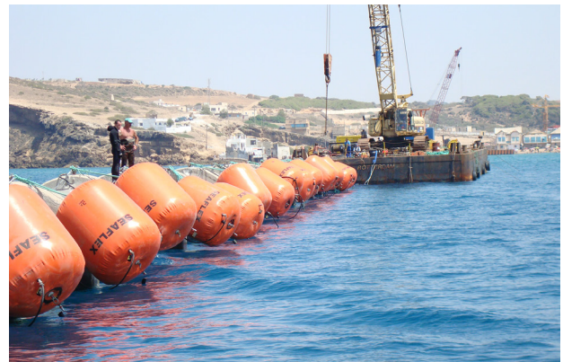
HDPE pipe is manoeuvred to the end of the previous string, where the MBUs are inflated before the pipe is flooded.
