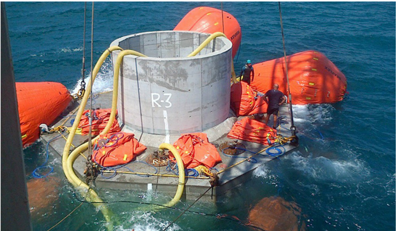
Sinking of Intake Tower (note submerged lower tier of FESAs, as upper tier is inflated)
