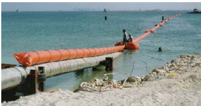
HIDD Pipeline, Bahrain, supported by Seaflex Kraken™ type 2650/2/13
